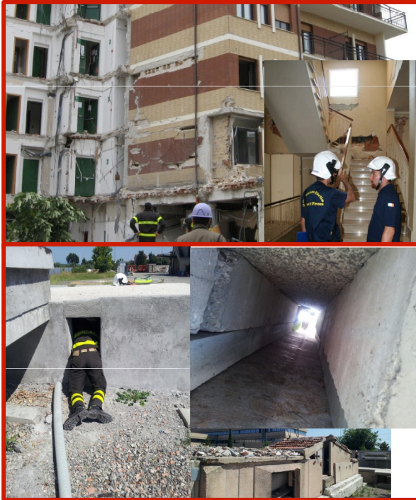
Entering and inspecting an unstable factory building after an earthquake event
